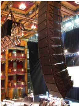
View Showing Arena Line Array
